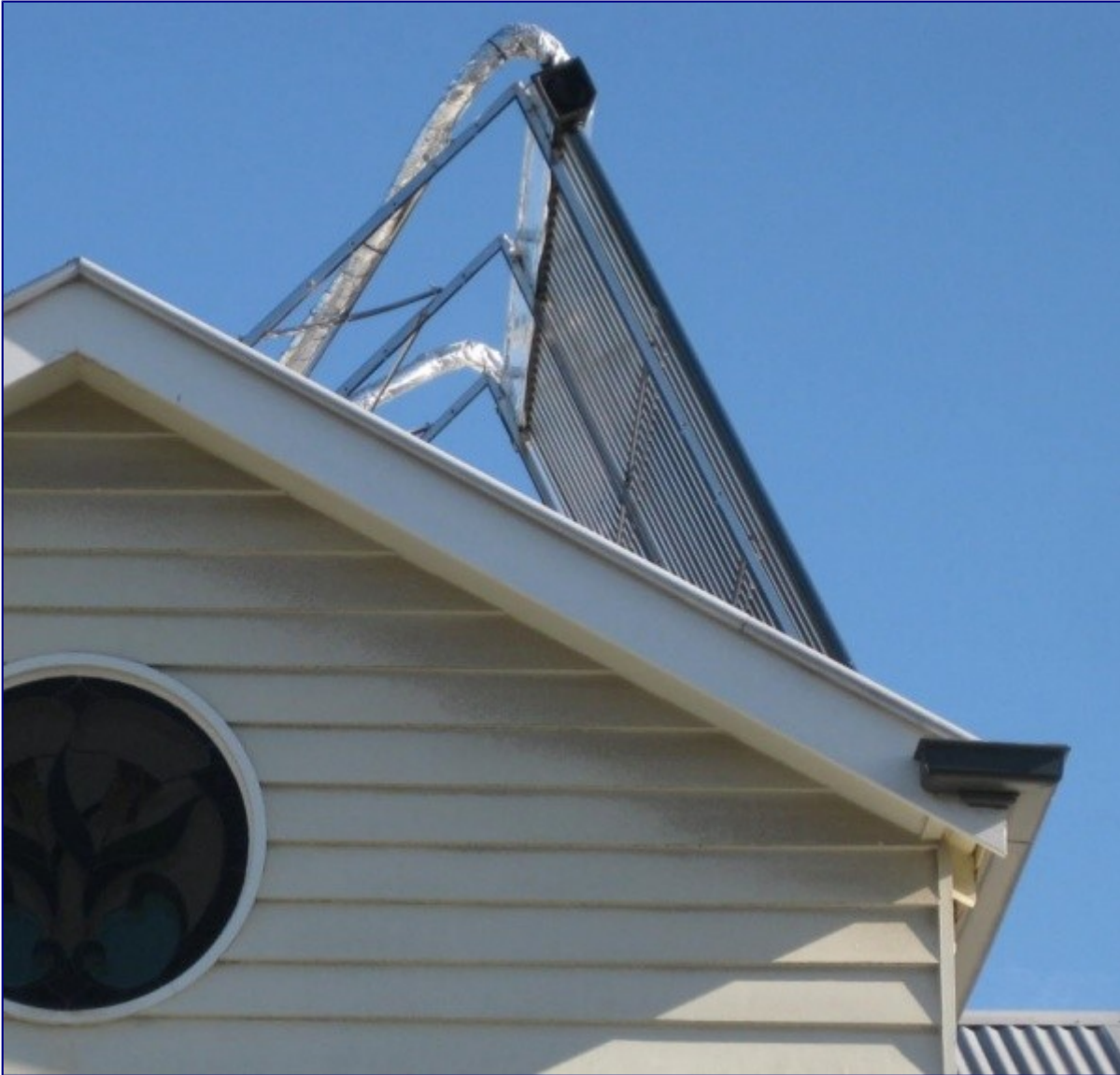
Figure A4.5: Evacuated-tube solar collector at 64° slope. Mid-day, mid-winter. Note shadow angle at right angle to face of collector
